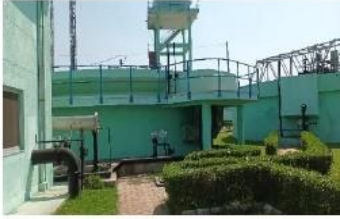
Image 7) Sludge digester along with gravity thickener
